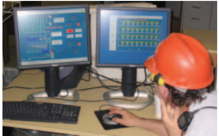
Twin displays are provided in the control room for easy access to information.
